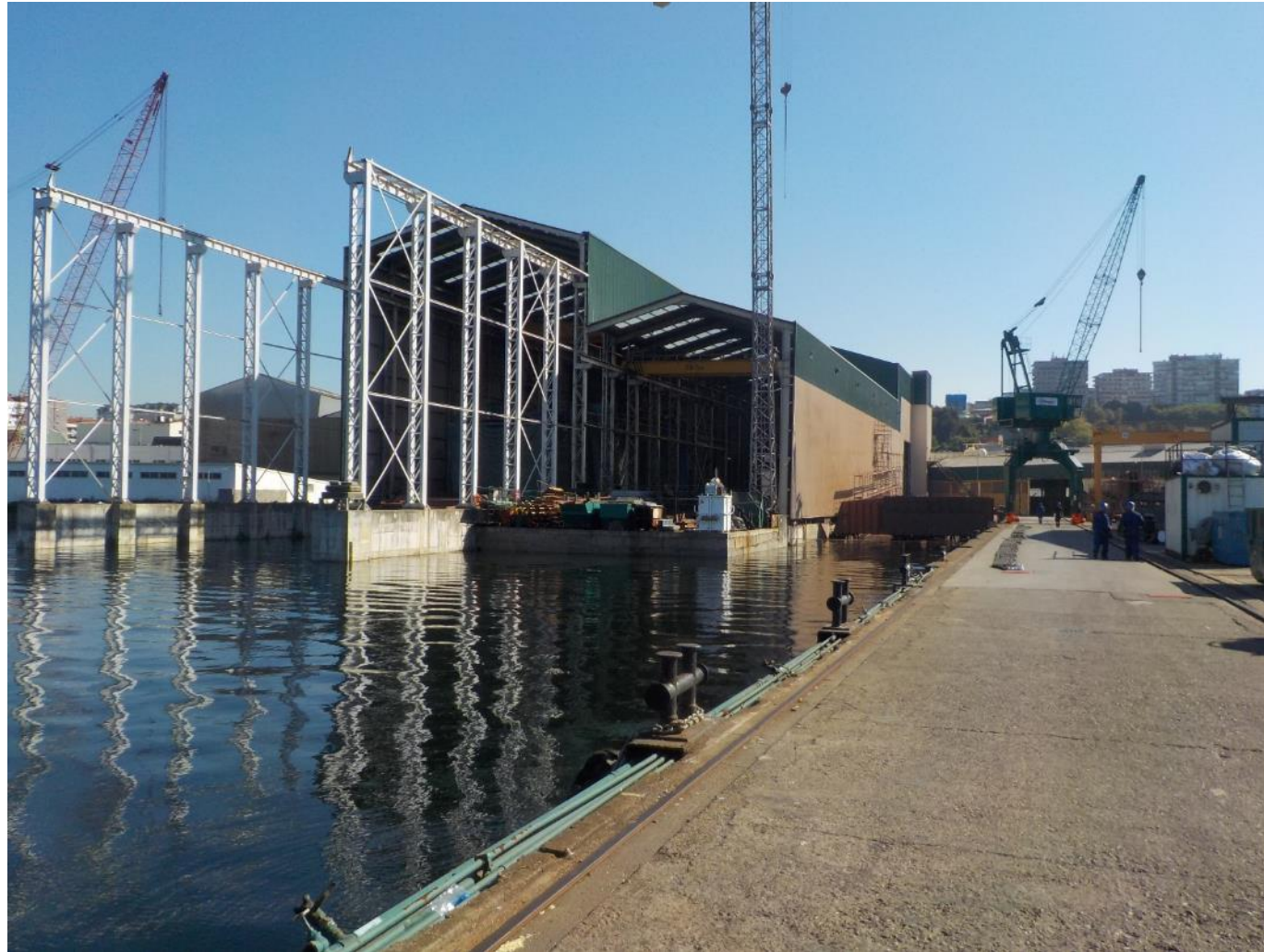
Welding hall at the shipyard where Svea is being built right now.
