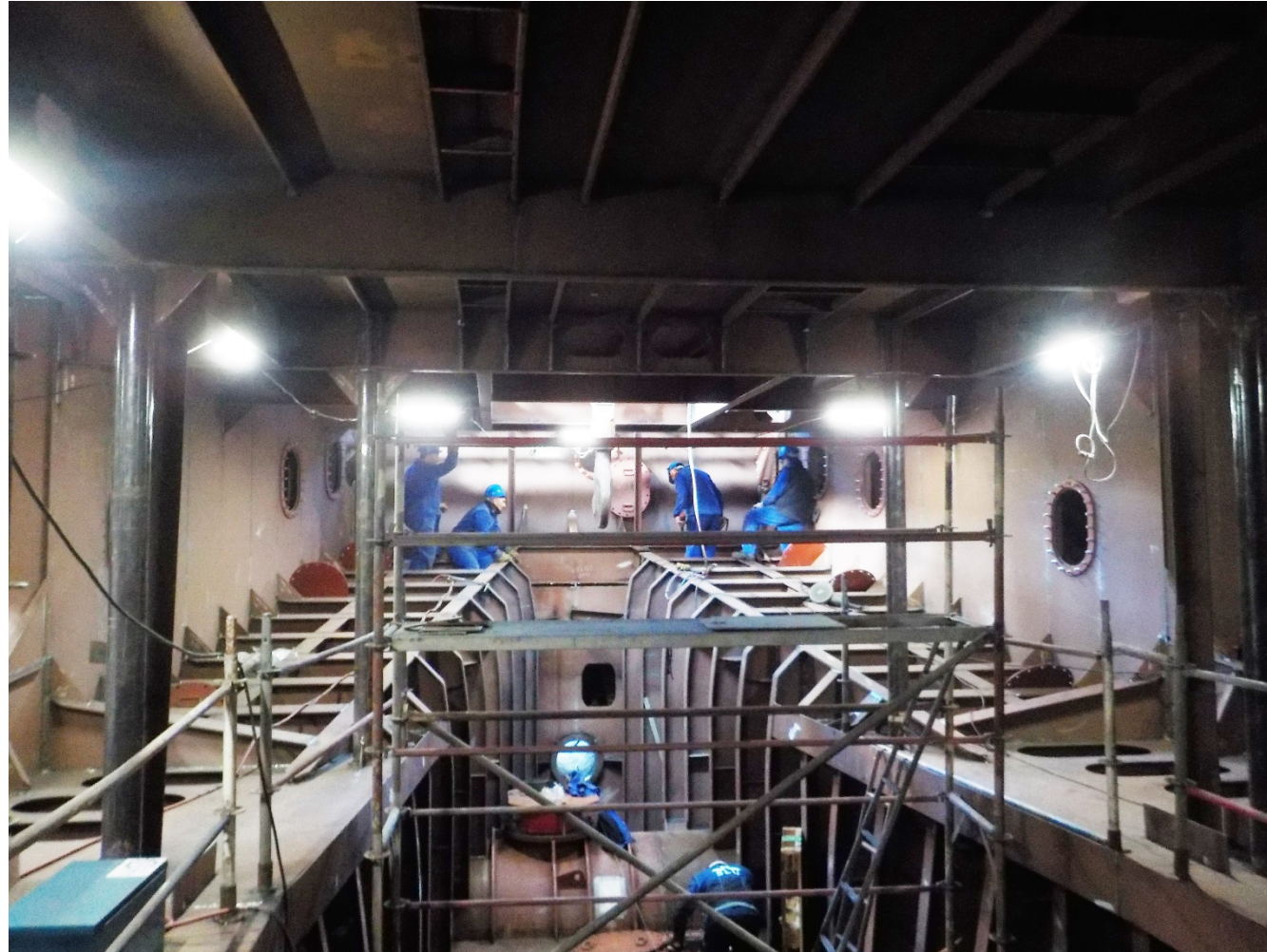
Here is the aft ship seen from the machinery space.
